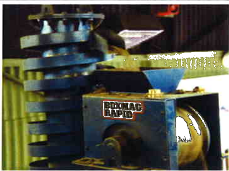
Fig 3 Spiral Lift Exit feeding Rotary Magnetic Separator
